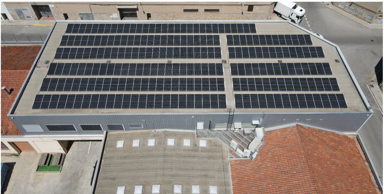
Aerial image of Lamp's rooftop with photovoltaic installation
